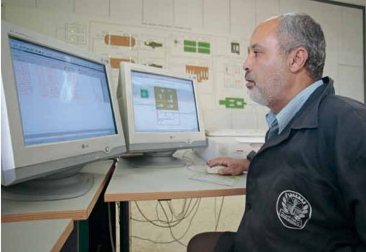
Employee at a sewage treatment plant working on a PC in a control room; November 2008, Jordan
